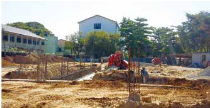
BEAP Project- On going construction of the fully integrated Accident and Emergency Trauma unit attached to Batticaloa Teaching Hospital
